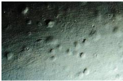
Osmotic blisters under the gelcoat
